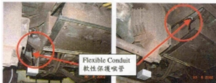
Photo 4 - Flexible Conduit and TDI Trip Switch Junction Box (After Modification) 相片四 - 軟性保護喉管和車鉤脫卡跳脫閘閘製連接盒(修改後)
