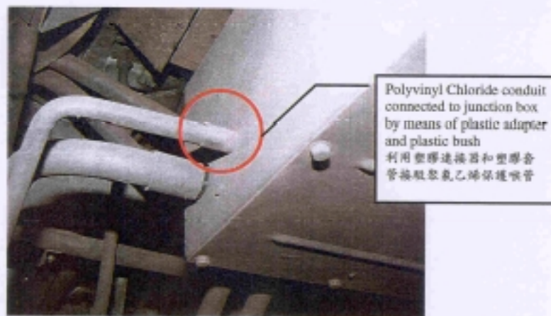
Photo 1 – TDI wiring connection (before modification)
