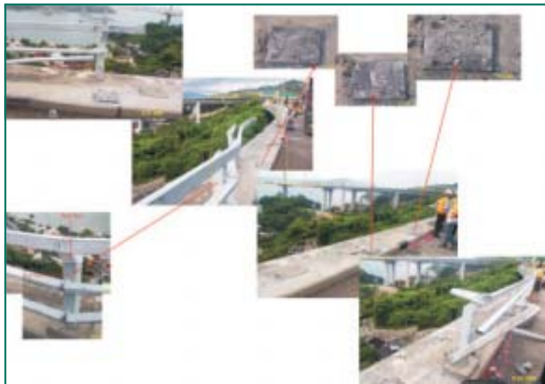
Figure 3.8 – The broken parapet
