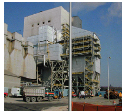
除氮設施/SCR
