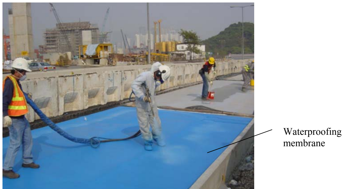
Figure 4 – Construction of trial panels of waterproofing systems under the Ngong Shuen Chau Viaduct Contract
