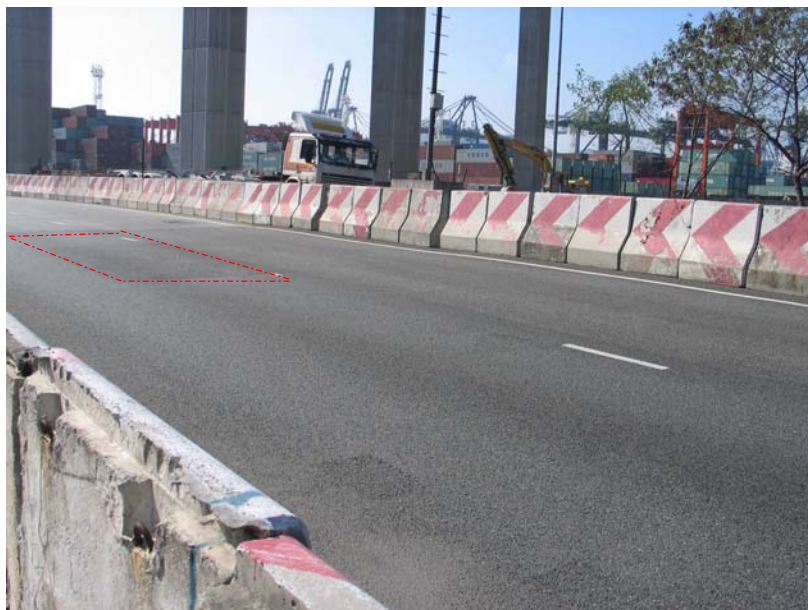
Figure 6 – Conditions of trial panels of waterproofing systems under the Ngong Shuen Chau Viaduct Contract. The red dotted line shows the repaired area of deformation that occurred at the thinnest panel of 50mm thick.
