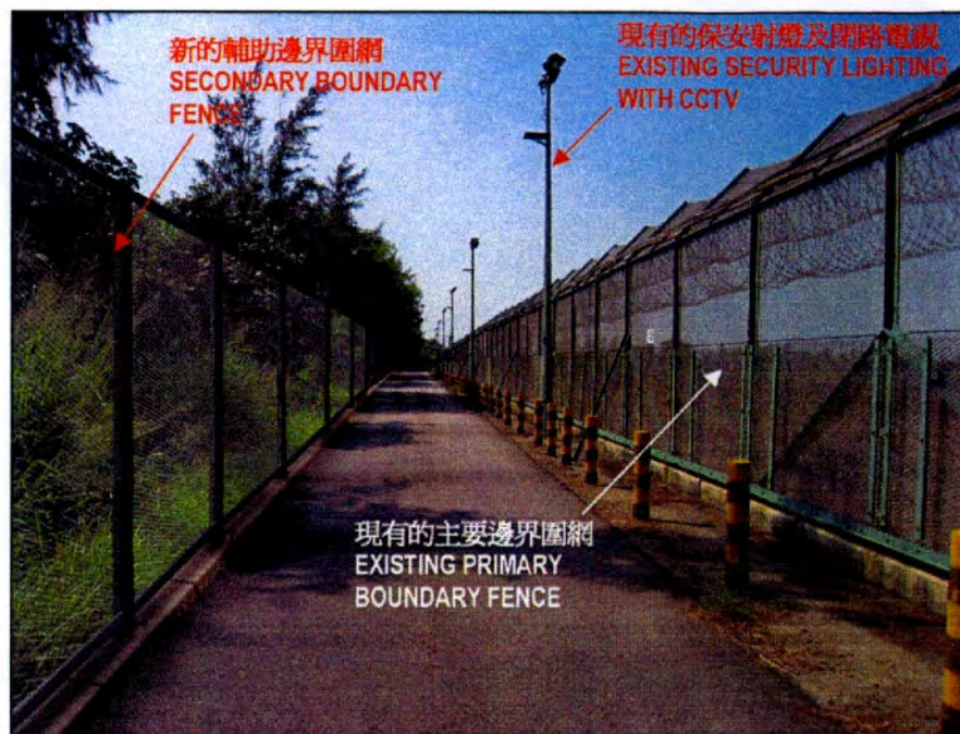
於現有巡邏通路以南興建的輔助邊界圍網 SECONDARY BOUNDARY FENCE TO BE CONSTRUCTED TO THE SOUTH OF EXISTING BOUNDARY PATROL ROAD
