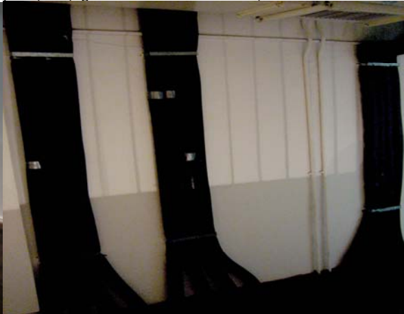
(fig. 4 Air-con drainage hosts without white box-cover)
