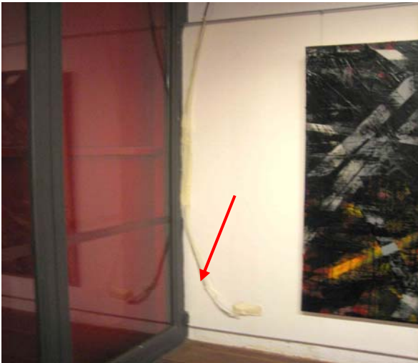
(fig. 7 Electricity lines running uncontrolled
