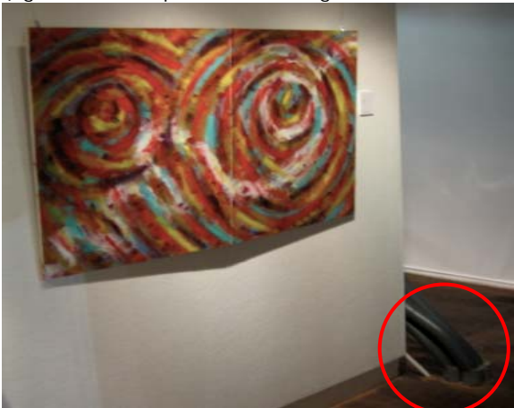
(fig 3. Exposed Air-con drainage hosts)
