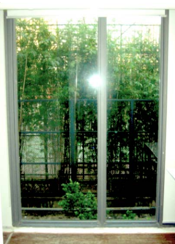
(fig. 7 UV infiltrated Door Window on 1/F Gallery)
