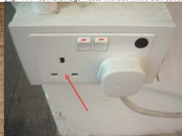
(fig.6 Exposed Unplugged Socket being turned on)
