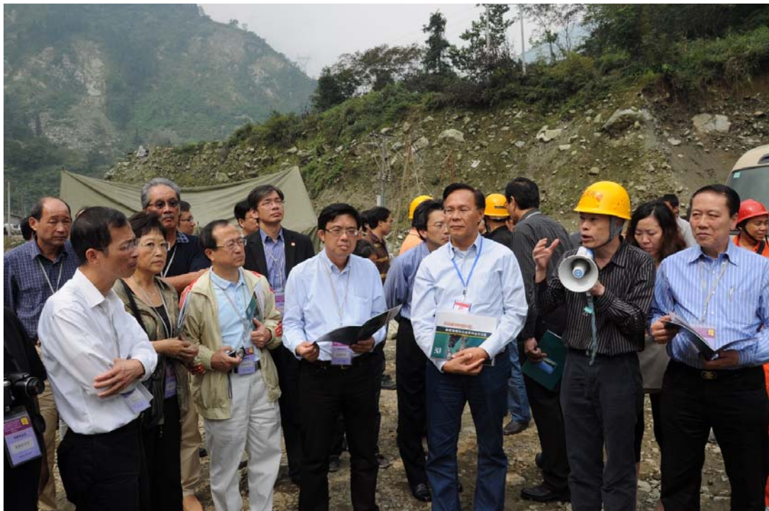
LegCo Members receive a briefing from an engineer on the progress of the construction work of the Provincial Road 303 Yingxiu to Wolong section.
