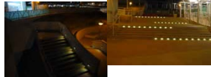
秀茂坪（南）邨戶外地方照明 External area illumination at Sau Mau Ping (South) Estate
