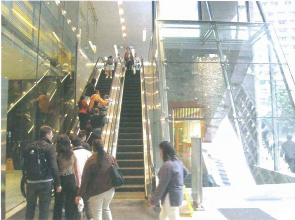
Photo 9.3: New escalator in the new building
