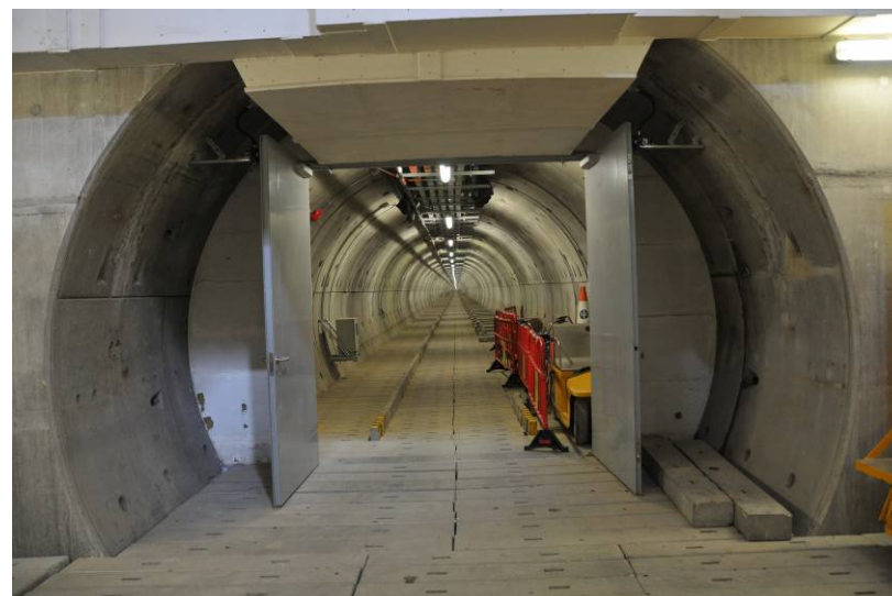
用以供電予機場及屯門區域的青山 電纜隧道 Castle Peak Cable Tunnel for the transmission cables supplying Airport/Tuen Mun area
