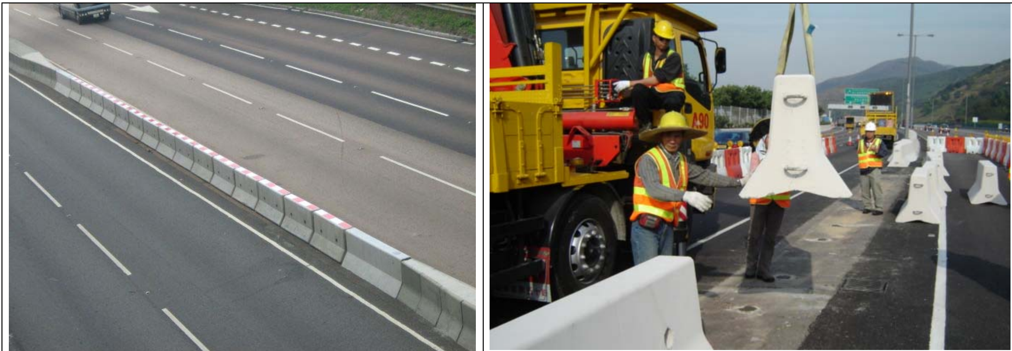
Figure 3: Removable Concrete Barriers
