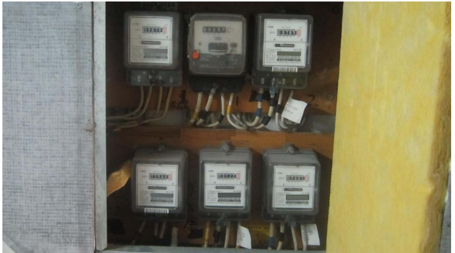
Electrical installations of the building
