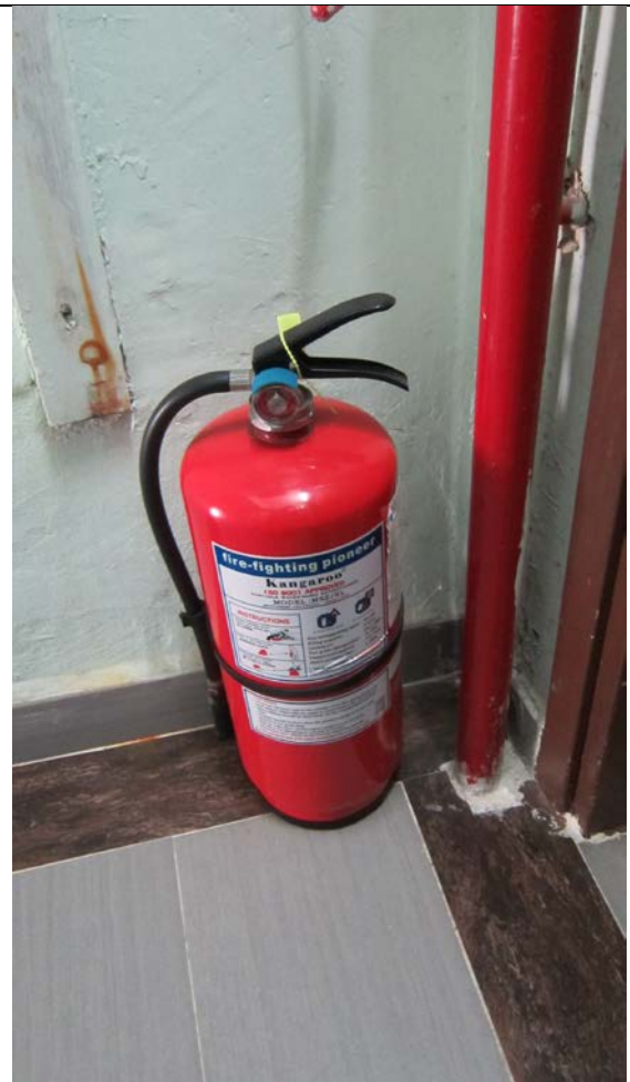
Fire services installation (fire extinguisher)
