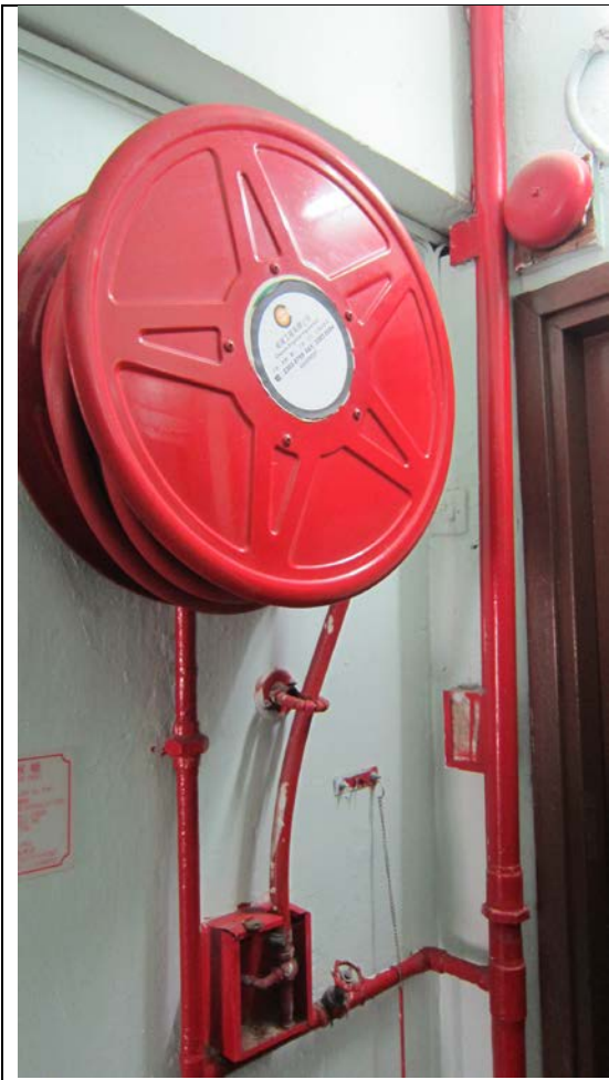
Fire services installation (hose reel)
