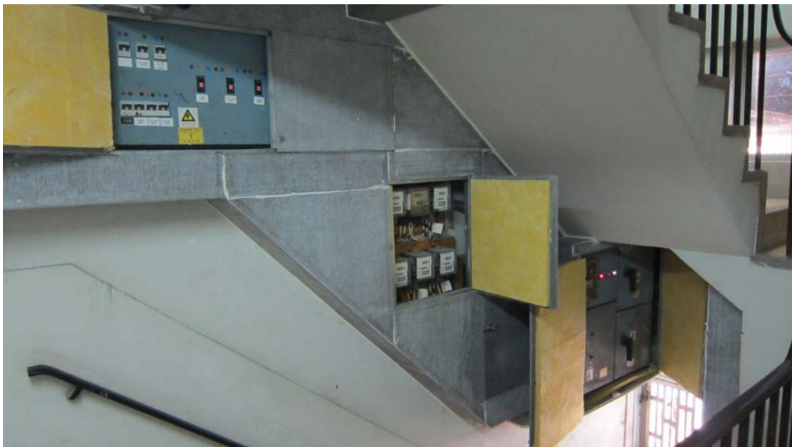
Certified distribution boxes and electric meters
