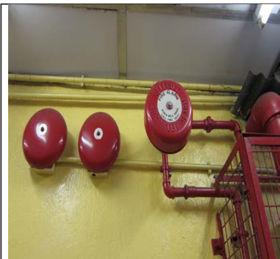
Fire services installation (fire alarm)
