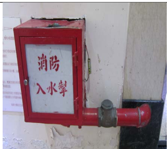
Fire services installation (fire services inlet)
