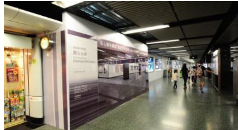
於鑽石山站內進行改建工程 Modification Works at Diamond Hill Station
