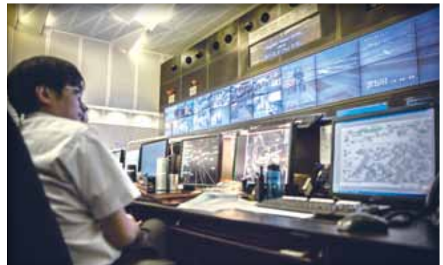
Operating 24 hours a day, the Integrated Airport Centre is at the heart of the airport's daily operational management.
