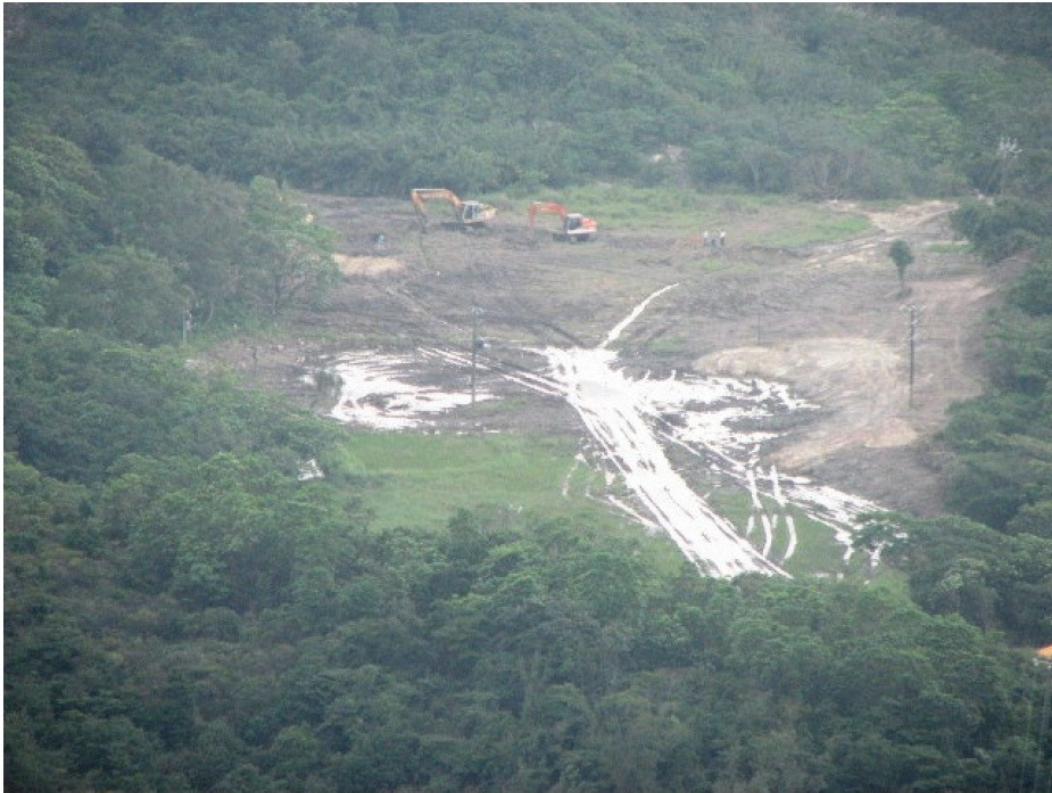
Figure 1 Excavation work in Tai Long Sai Wan in 2010 (Photo taken on Jun 2010)
