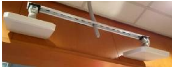
RFID Reader Installed at Checkpoints
