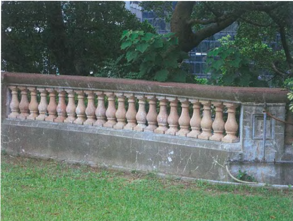
E.16 Balustrade at north end of Flagstaff House garden, at crest of slope above Queensway.
