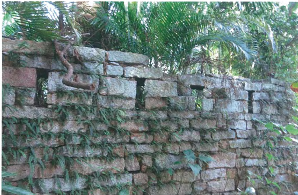
E.7 View from outside, of group of four generally north- east facing loopholes for firing in the historic defensive squared rubble masonry wall.
