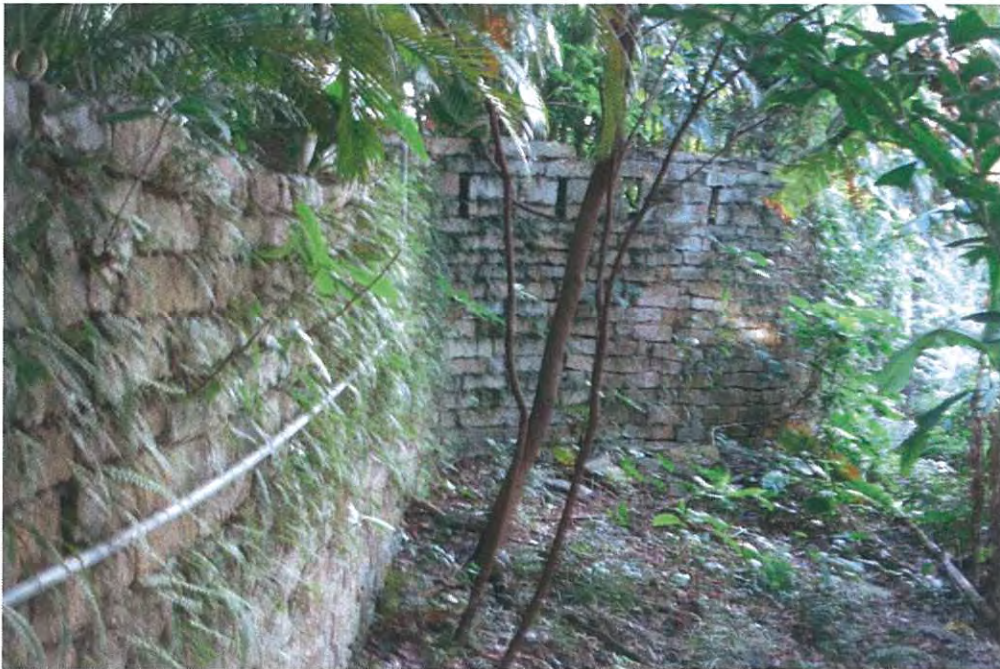
E.10 View looking south along historic rubble masonry wall flanking the north-western side of the Flagstaff House garden area, which would have been protected by the four loopholes which can be seen in the part of the wall ahead.
