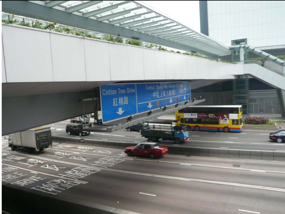
Gantry sign lighting
