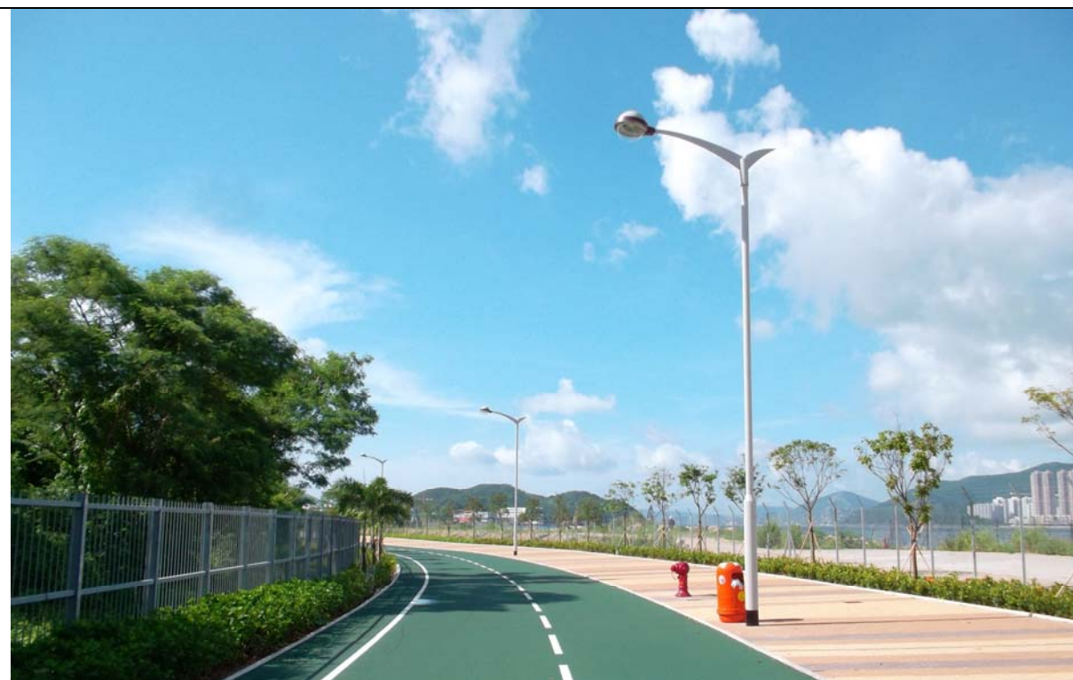
Cycle track lighting
