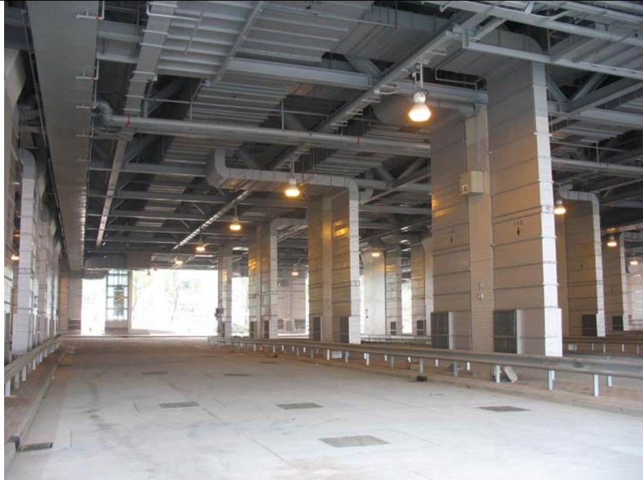
Highbay lighting at public transport interchanges
