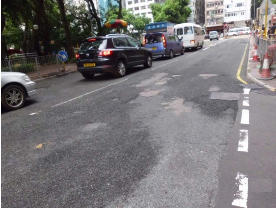
Figure 1: Pavement condition before repair works
