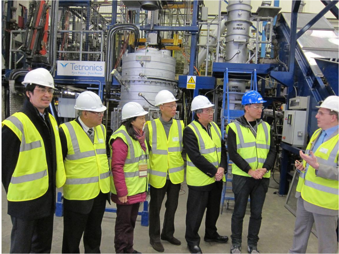
Members of the delegation receive a briefing on the operation of the Swindon Gasification Plant. (Second from left: Hon WONG Ting-kwong, Dr Hon Elizabeth QUAT, Mr WONG Kam-sing, the Secretary for the Environment, Ir Dr Hon LO Wai-kwok and Hon Paul TSE Wai-chun)
