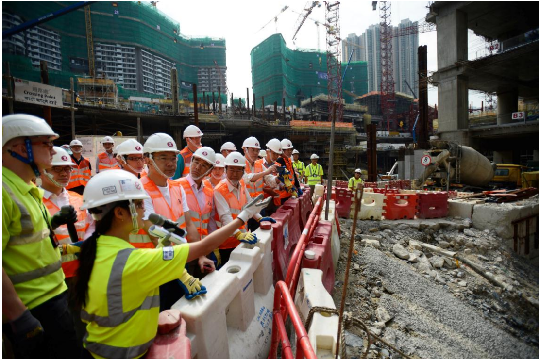
Members observe the construction site of the WKT of the Hong Kong Section of the XRL.
