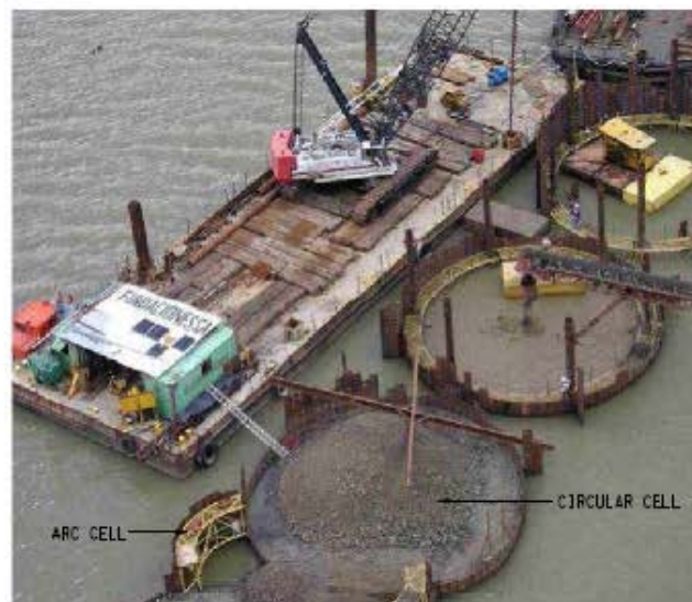
C. CONSTRUCTION OF ARC CELL CONNECTING TWO CIRCULAR CELLS 建造弧形圍堰以連接圓環式圍堰
