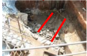
7) 石砌路徑及前馬頭涌河岸的石結構 Stone footpath and stone structure which forms the riverbanks of the former Ma Tau Chung (原址保留 Preserve in-situ )
