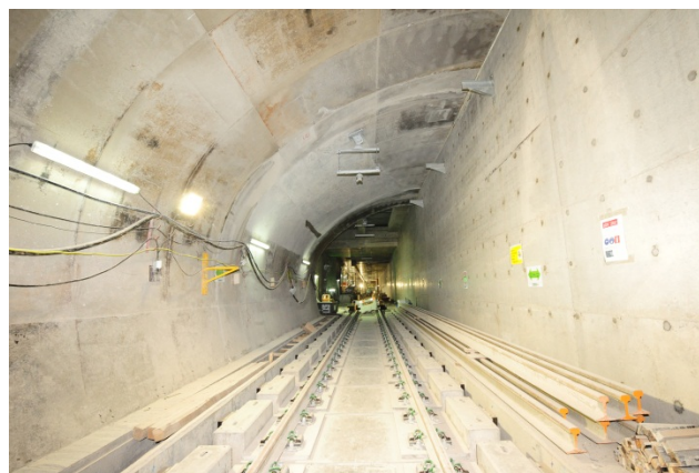
Track works at tunnel between Yau Ma Tei and Ho Man Tin
