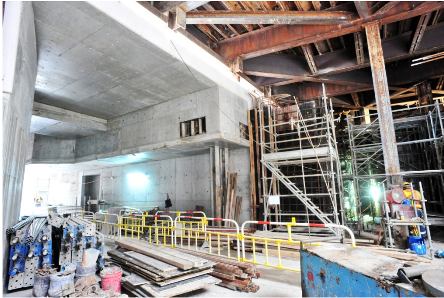
Station structural works in progress under the temporary traffic deck at South Horizons
