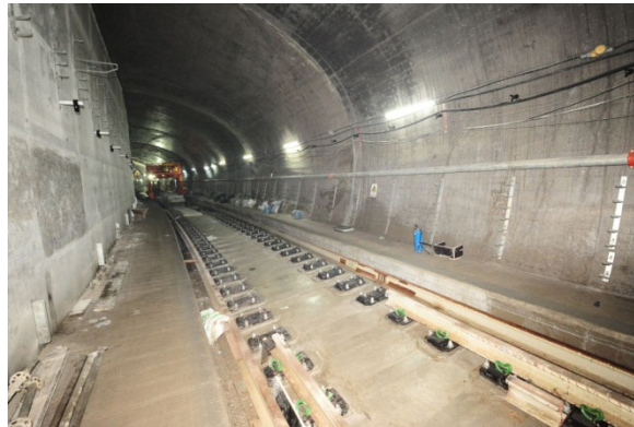
Structural works of railway tunnels between Yau Ma Tei and Ho Man Tin
