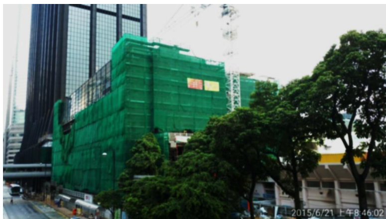
The re-provisioned Wan Chai Swimming Pool is expected to complete by end of 2015
