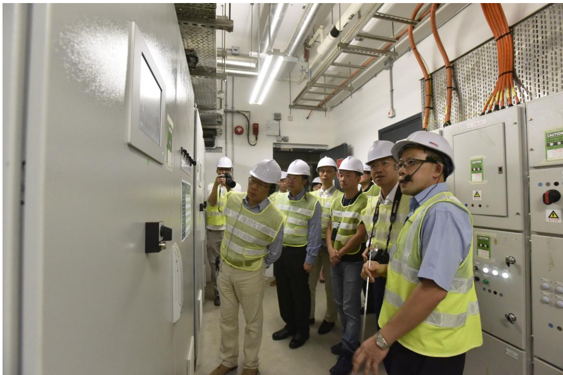
Members of the Legislative Council visit the Continuous Emission Monitoring System Room in the Sludge Treatment Facility in Tuen Mun.
