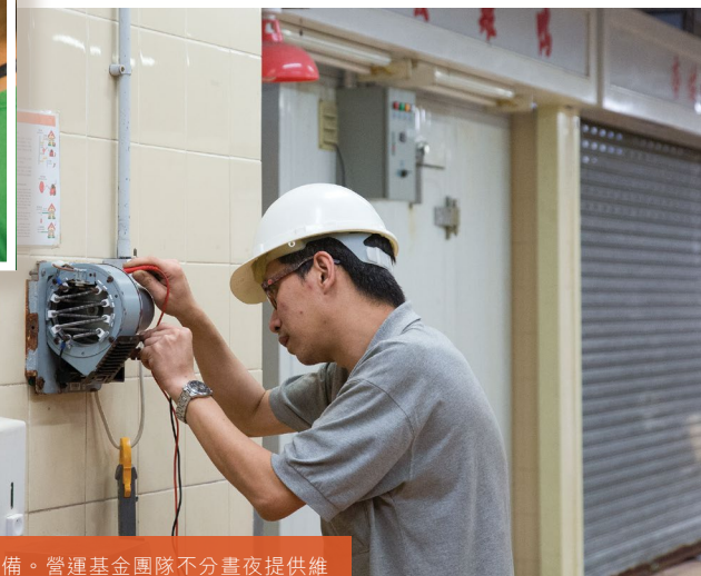
員工於西營盤正街街市維修機電設備。營運基金團隊不分晝夜提供維修保養服務，讓市民享用可靠、方便的市政設施。 Staff repairing E&M equipment at Centre Street Market in Sai Ying Pun, one of the many services the EMSTF team provides round the clock to make municipal facilities reliable and convenient to users.
