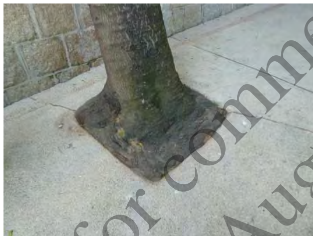
Fig. 6 A bad example showing a tree surrounded by concrete around the root collar
