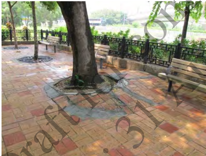
Fig. 2 Pavement lifting caused by root growth
