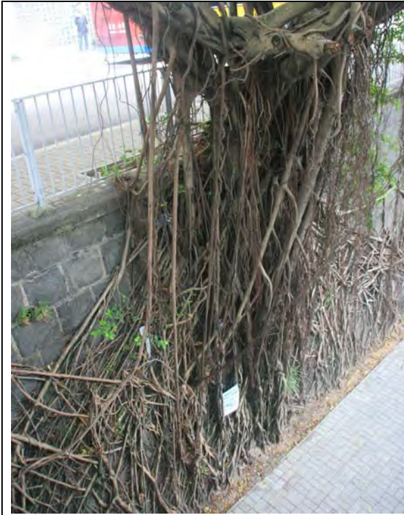
Photo No. 6 – Provision of rooting areas at the toe of the retaining wall
