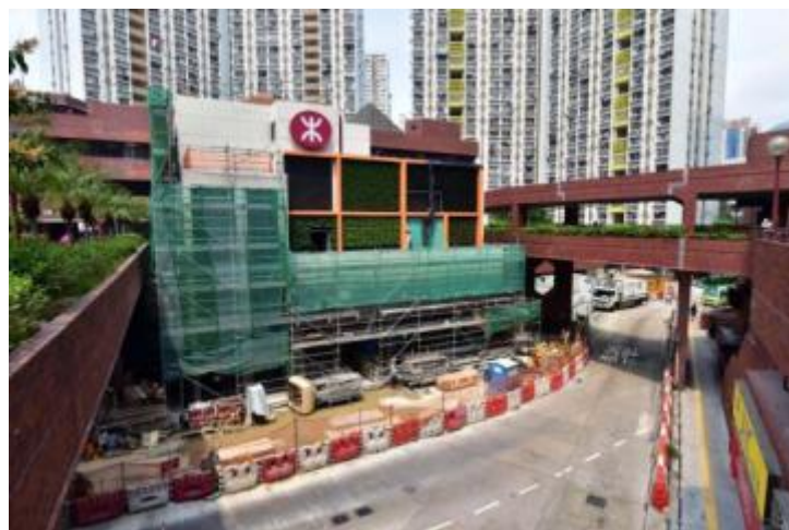
Above-ground structural works of Lei Tung Station Entrance B have been completed
