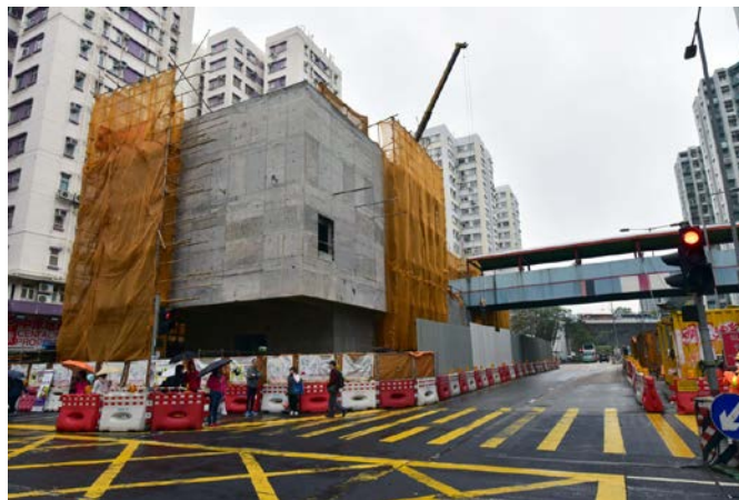
The external finishing work of the entrance at Man Siu Street is in progress.
