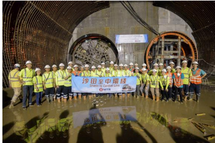
Tunnel breakthrough of TBM tunnel from Diamond Hill to Ma Chai Hang
