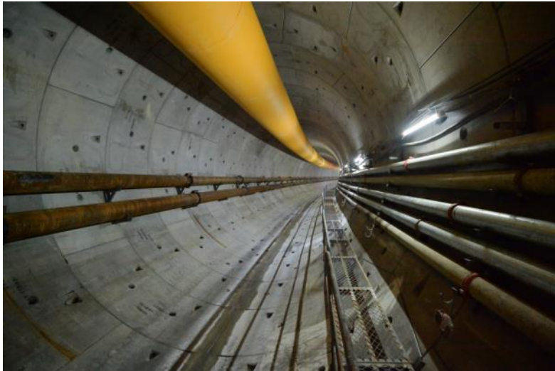
Excavation of the up-track tunnel between CBTS and Exhibition Station was completed
