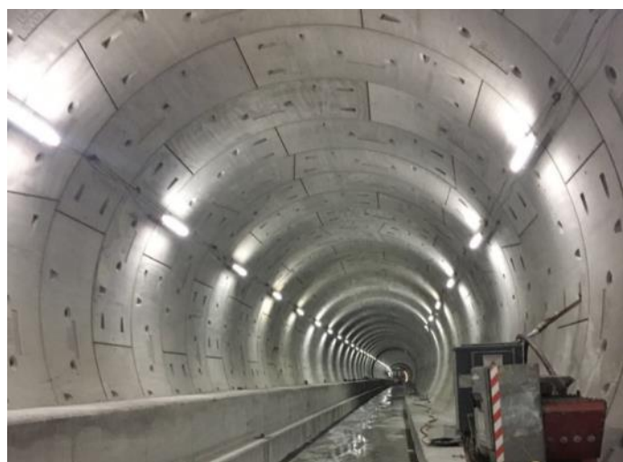
Internal structural works at down-track tunnel from Diamond Hill to Ma Chai Hang
