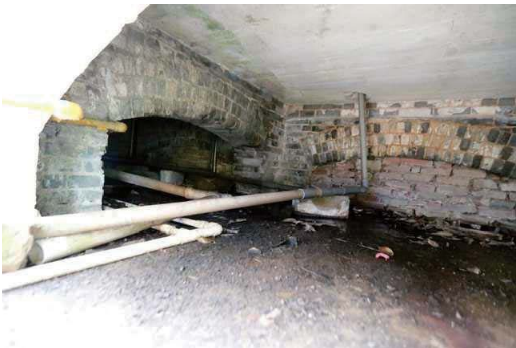
Typical view of the ventilated sub-floor, showing grey brickwork and arched supports to the main ground floor structure above.
