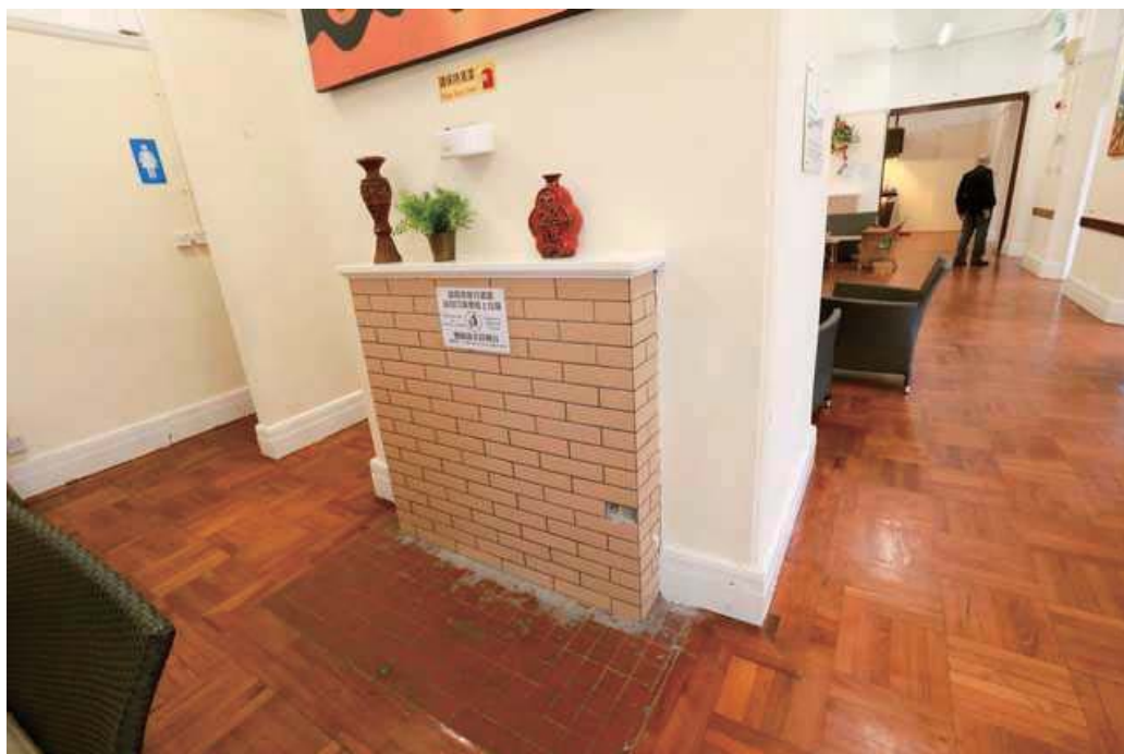
Brick chimney breast with fireplace is now bricked up. A portion of old ceramic red quarry tile flooring still remains.
