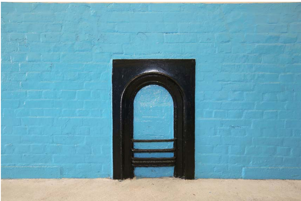
A cast iron fireplace in a smaller room on the first floor, originally used for senior soldiers' accommodation.
