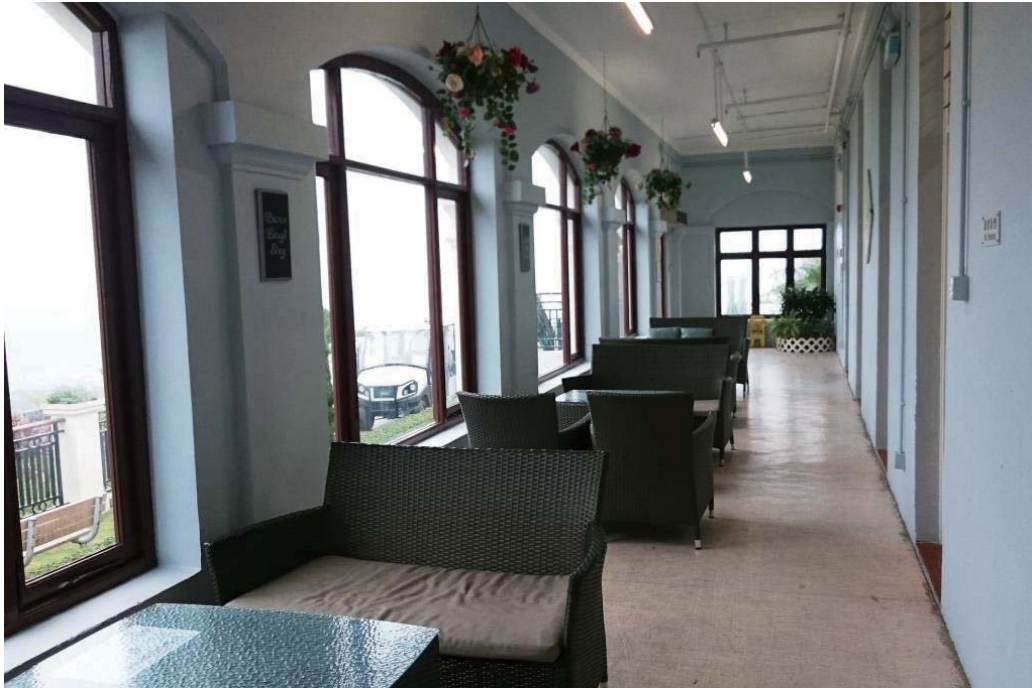
The front verandah with windows installed. Originally the open verandah would have been a common sitting-out area for the tenants.
