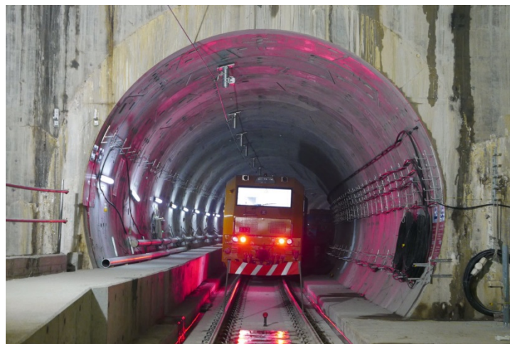
Trackside auxiliary works are on-going at the tunnels from Kai Tak to Diamond Hill
