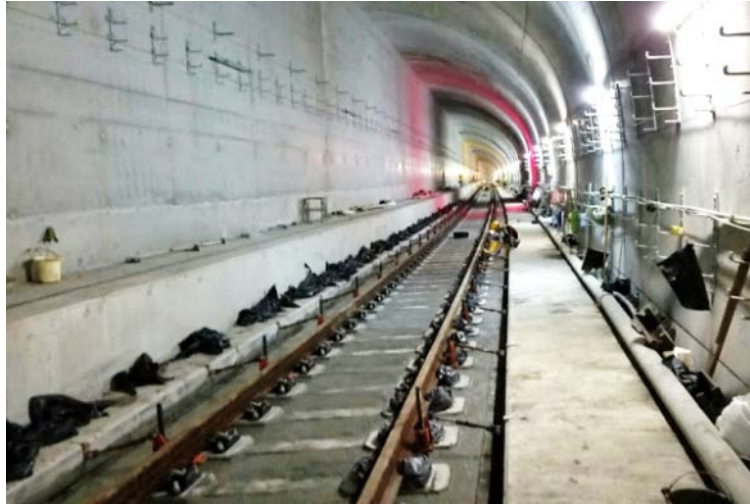
Track works for the TBM tunnels from Diamond Hill to Ma Chai Hang
