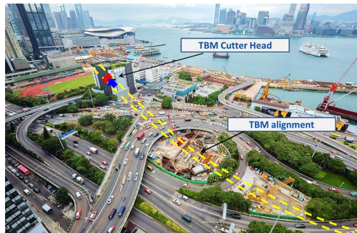
Excavation of the down-track tunnel between CBTS and Exhibition Station was completed
