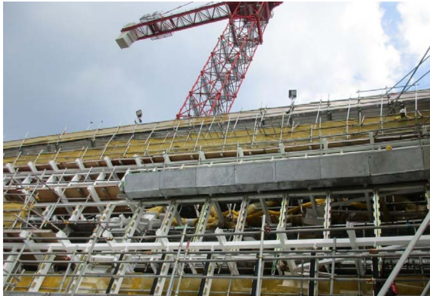
Installation of sub-frames for glazing and aluminum panels at the western side of the Station Entrance Building
