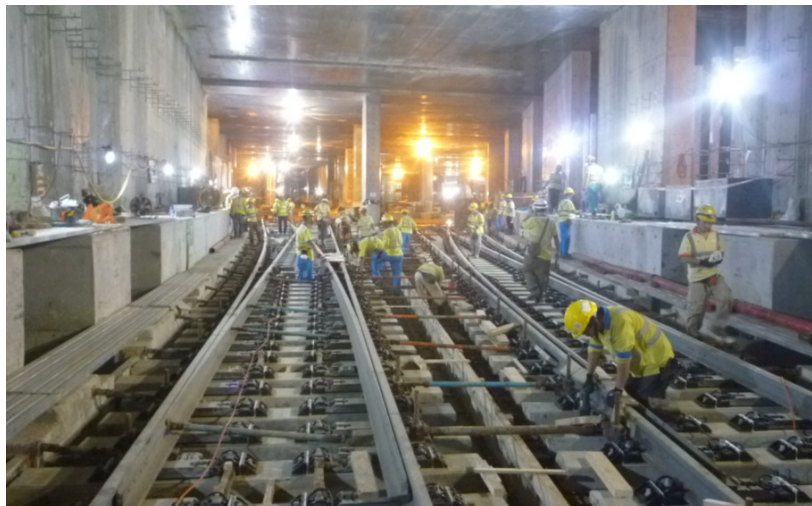
Track and turnout installation at the southern section of the approach tunnels is in progress
