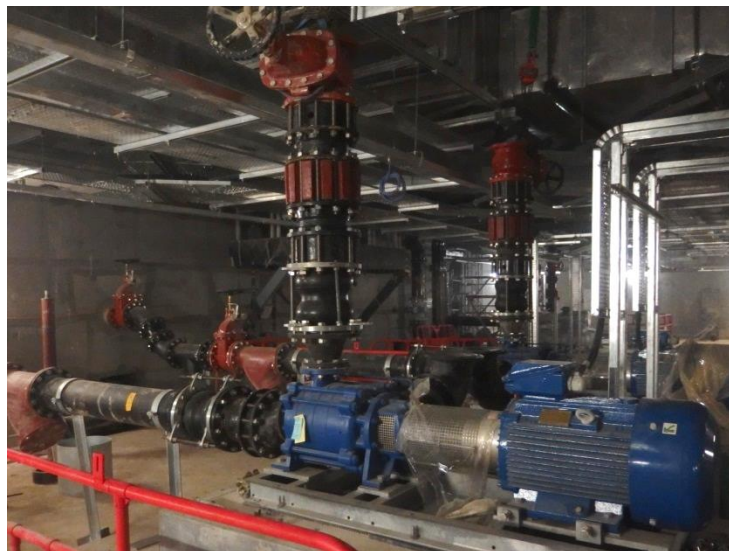
Fire services plumbing & drainage systems in the pump room at WKT Level B3
