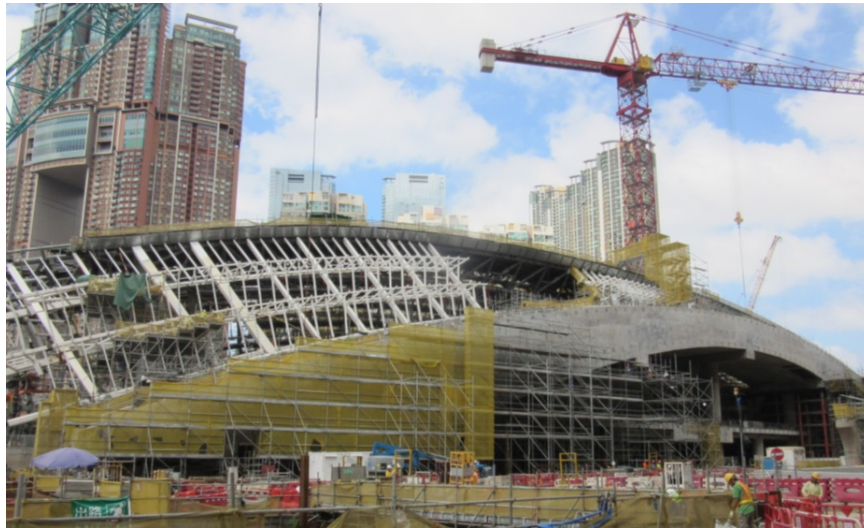
Erection of secondary and tertiary steel members at the eastern side of the Station Entrance Building
