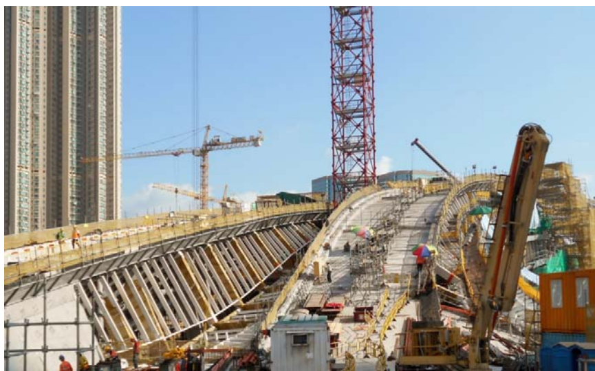
Completion of roof trusses concreting at the northern side of the Station Entrance Building
