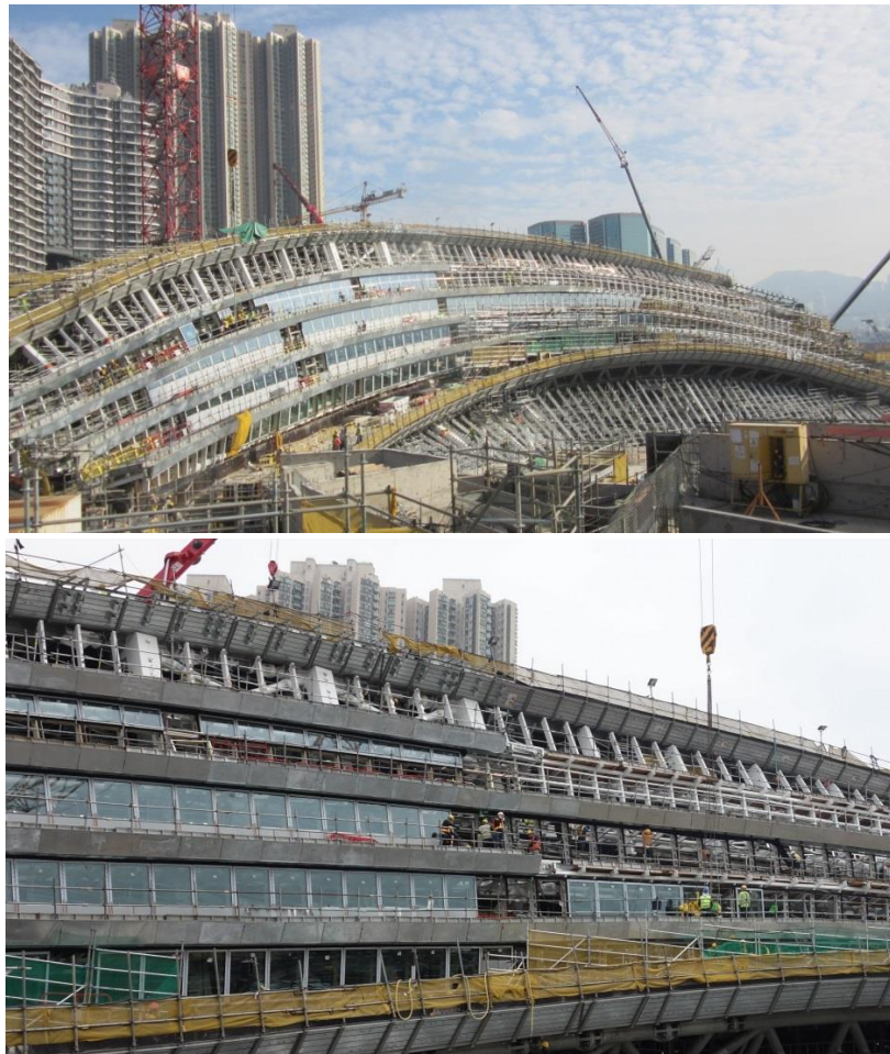
Installation of glazing panels at the western side of the Station Entrance Building
