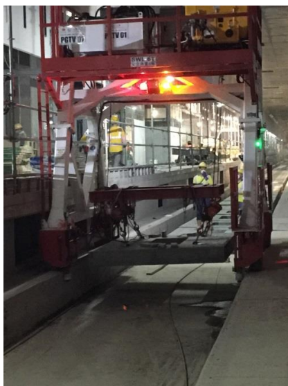
Special lifting gantry for laying the precast slabs at WKT North platform level
