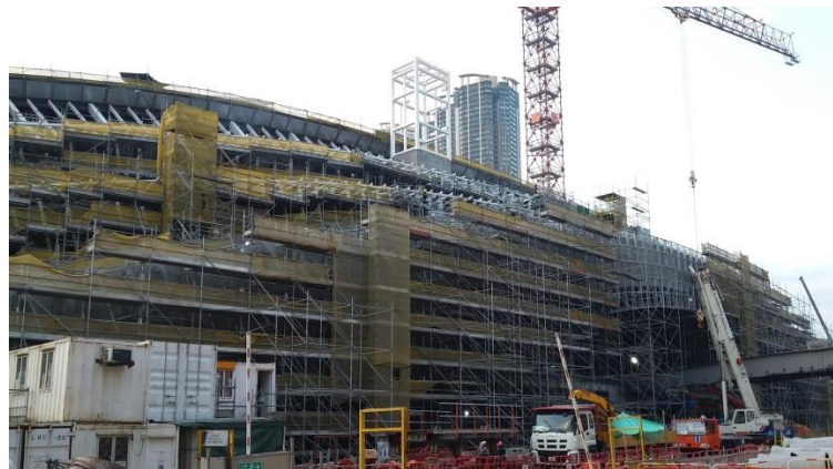
Erection of lift, secondary and tertiary steel members at the eastern side of the Station Entrance Building
