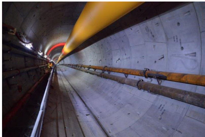
Excavation of the up-track and down-track tunnel between CBTS and Exhibition Station are completed
