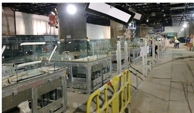
Installation of immigration counters in the Hong Kong Customs, Immigration and Quarantine areas at WKT Level B3
