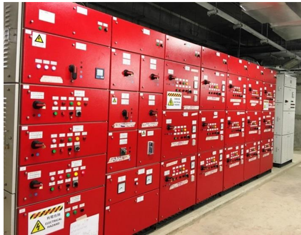
Energization of Motor Control Centre at WKT South
