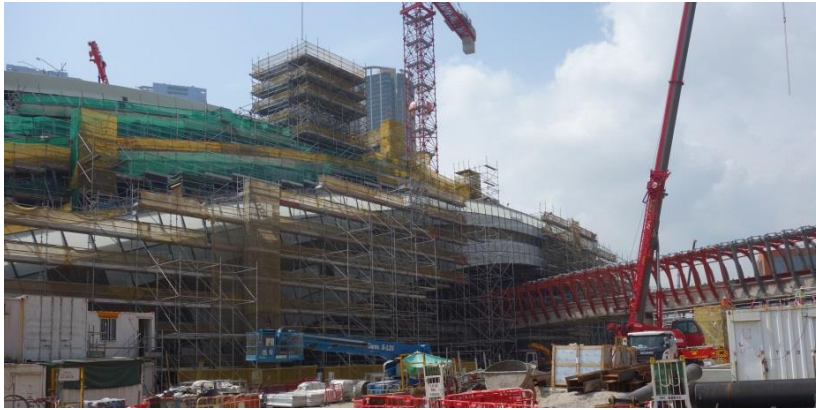
External Wall System installation at the eastern side of the Station Entrance Building
