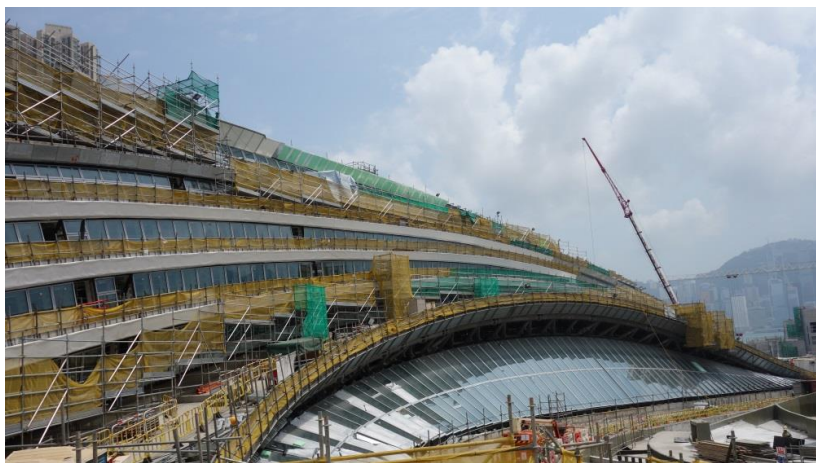
Installation of glazing panels at the western side of the Station Entrance Building
