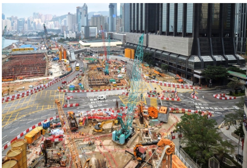
The junction between Convention Avenue, Fleming Road and Expo Drive East will be shifted eastward in phases
