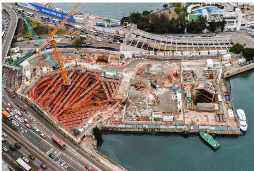
Excavation of the ventilation facilities at the former Police Officers' Club works site
