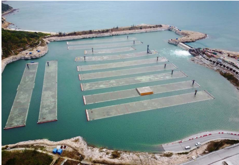
IMT casting yard is being re-watered to float the tunnel units and prepare for immersion in Victoria Harbour
