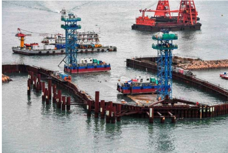
The first IMT unit is successfully immersed onto the seabed of Victor Harbour (This photo captured the first immersed tube tunnel during immersion)
