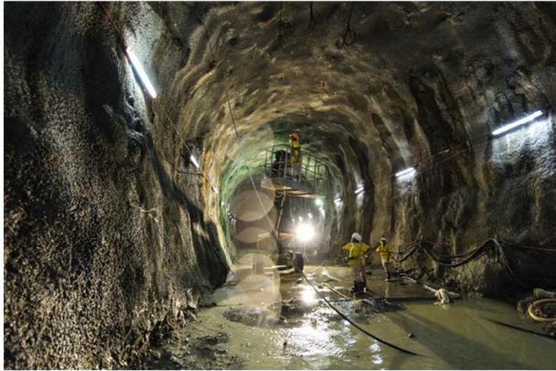
SCL overrun tunnel was completed by drill and blast method in June 2017
