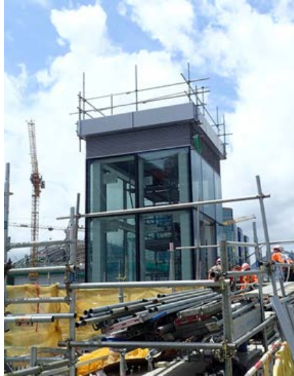
Installation of lift at the roof top at the eastern side of the Station Entrance Building
