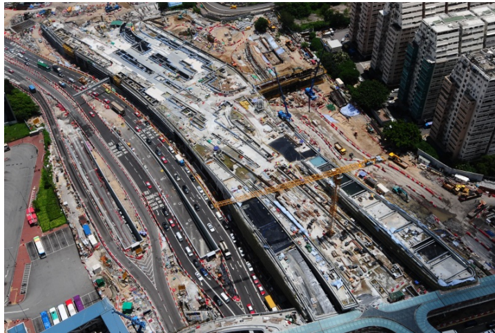
The construction of the West Kowloon Station Bus Terminus near Jordan Road is progressing
