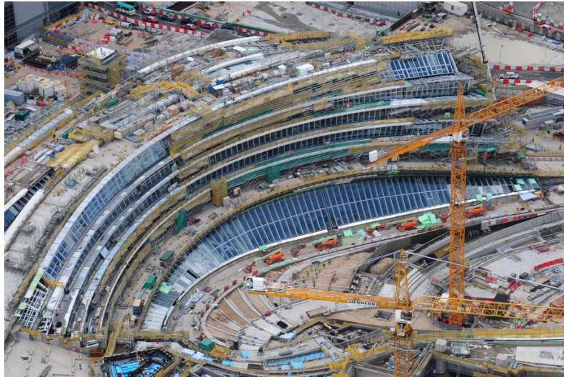
Installation of glazing panels at the western side of the Station Entrance Building
