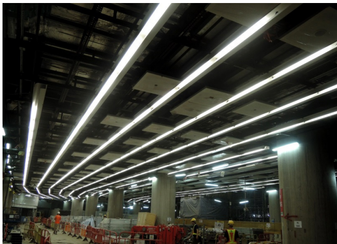
Lighting of the arrival hall at the Station is powered on
