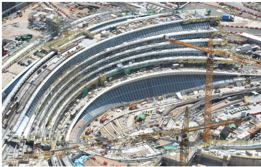
Weather-tightness for the main roof of the Station Entrance Building has been achieved
