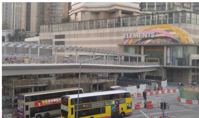
One of the footbridges at the western side of the Station connecting to Kowloon Station and nearby locations
