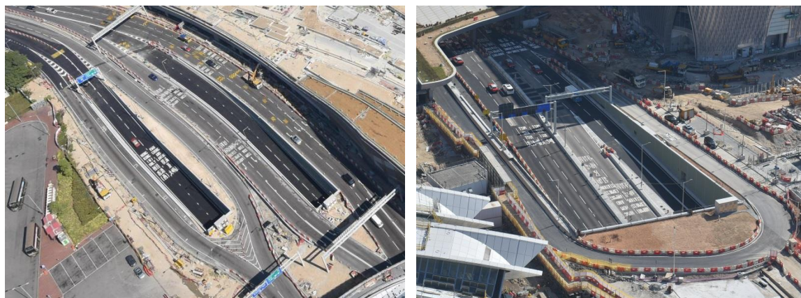
Stage 2 opening of the Lin Cheung Road / Austin Road West Underpass has been implemented
