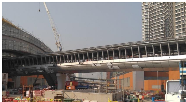
One of the footbridges at the eastern side of the Station connecting to Austin Station
