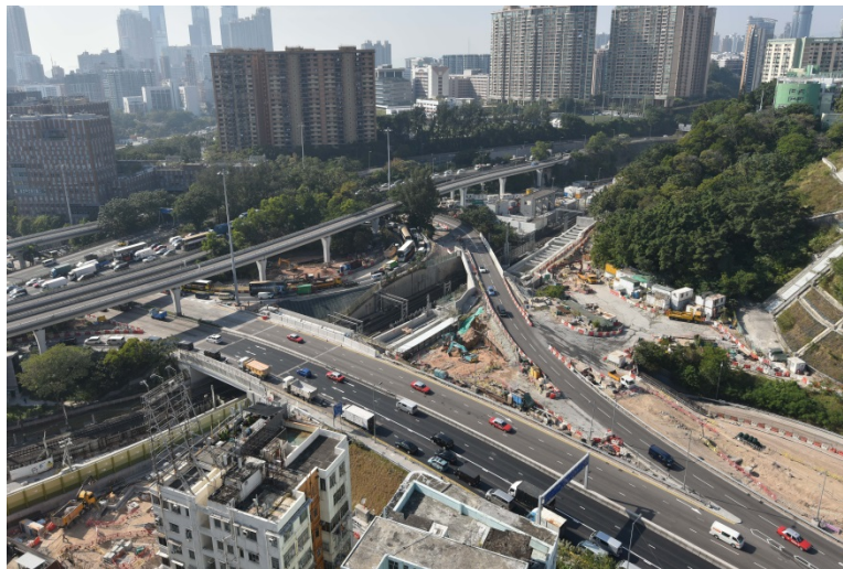
Temporary Traffic Management Schemes completed along Chatham Road North, Winslow Street underpass slip road and Hong Chong Road slip road
