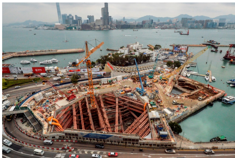
Excavation of the tunnel ventilation facilities at the former Police Officers' Club works site
