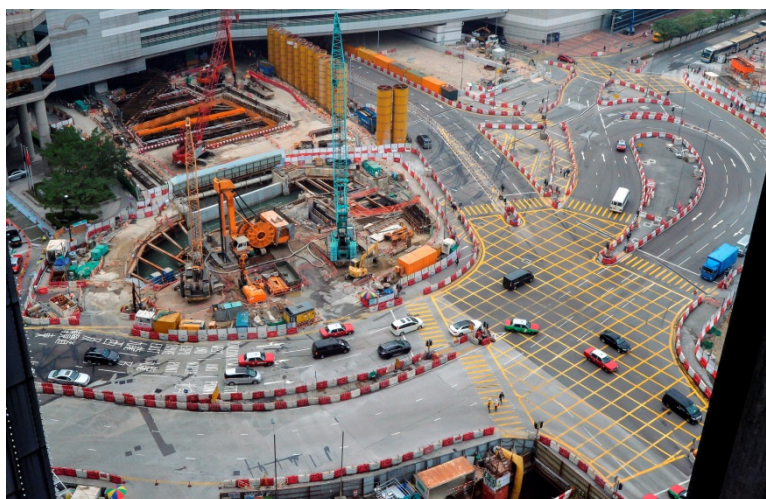
Temporary traffic management schemes are being implemented in phases in Wan Chai North
