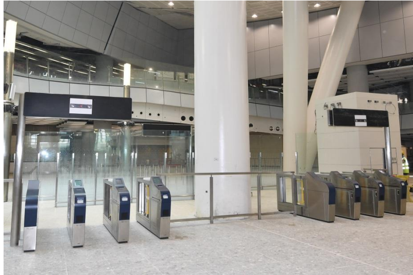
Ticket gates have been installed at Hong Kong West Kowloon Station
