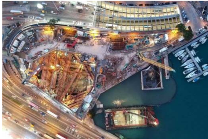
Excavation of the tunnel ventilation building at the former Police Officers' Club works site
