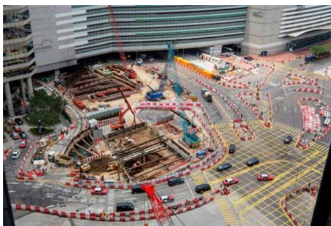
Temporary traffic management schemes are being implemented in phases in Wan Chai North
