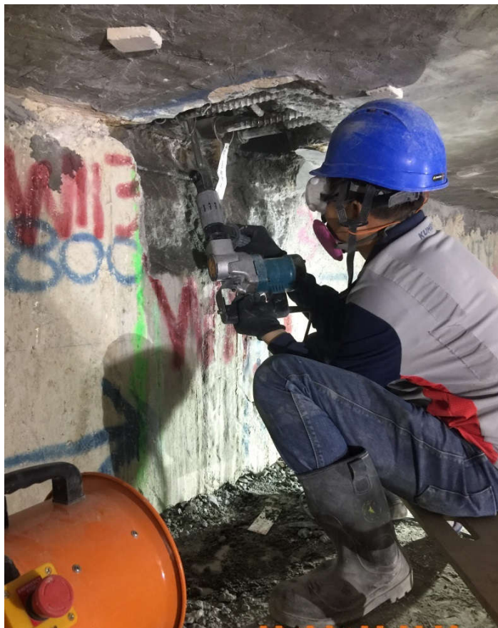
開鑿石屎以露出鋼筋及螺絲帽 Open up concrete to expose couplers and steel bars
