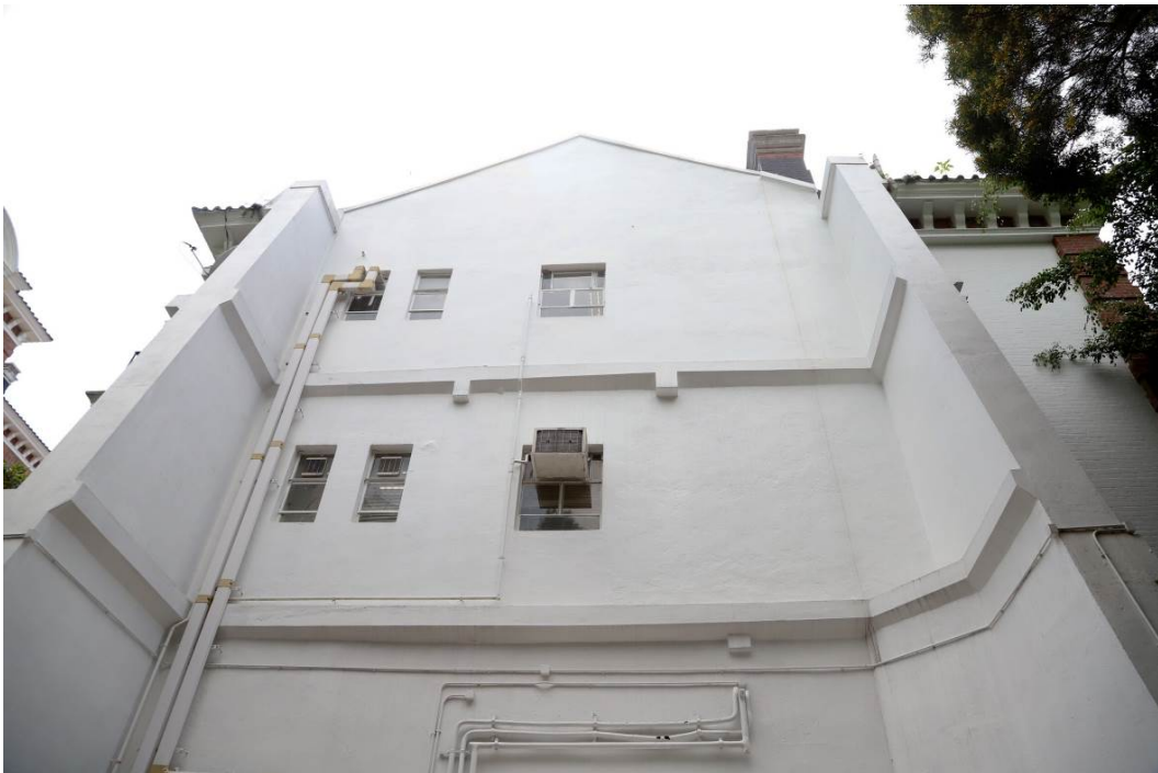
Two buttresses were erected at the collapsed portion after the severe landslide in 1966
