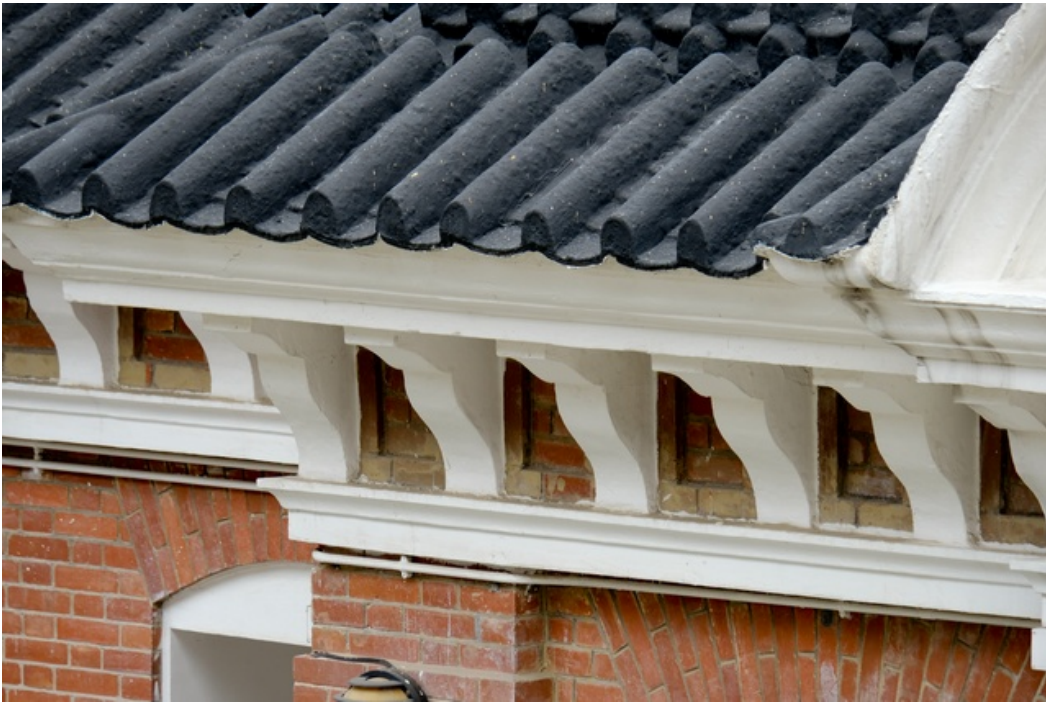
The roof eaves with numerous supporting brackets as a design feature and a moulded cornice underneath
