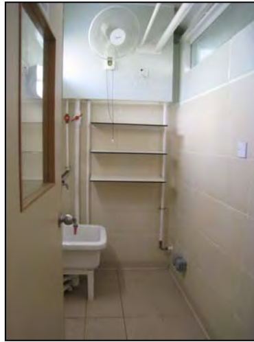
Slop sink and storage facilities inside a compartment
