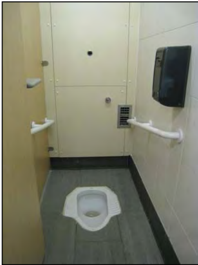
Cistern and related piping are concealed from view, leaving the toilet cubicle clean and tidy
