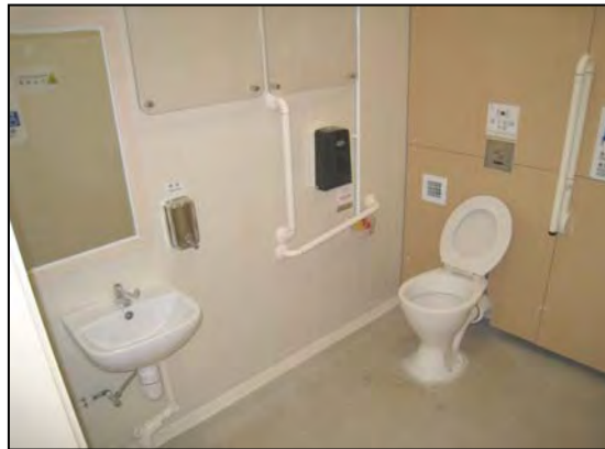
Tai Po Centre Public Toilet (Tai Po)
