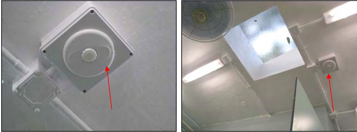
Motion sensor control installed inside toilet
