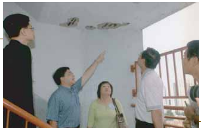
Members examined defects in the ceiling of a flat in the Chuk Yuen North Estate, which were sold to tenants under the Tenants Purchase Scheme in which the authority promised a seven-year structural safety guarantee for its maintenance.
